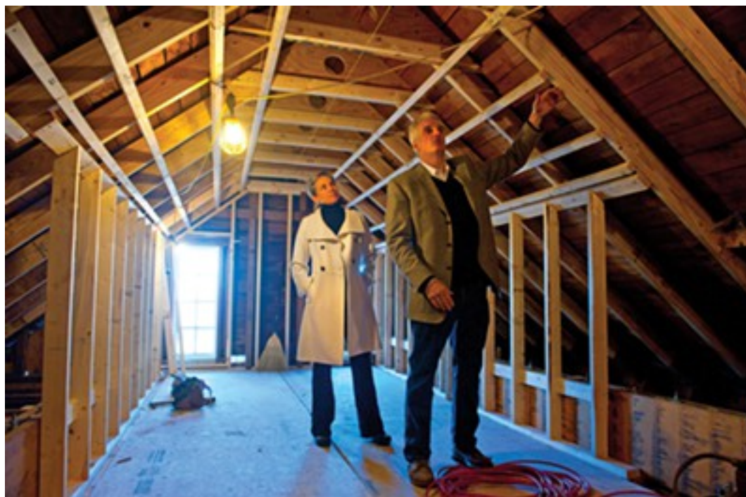
Scott Elmquist Paul and Julie Weissend inspect renovation progress on the third floor of Goshen, a historic Gloucester County farmhouse that dates to 1750 and where the overall project includes the drilling of geo-thermal wells.
